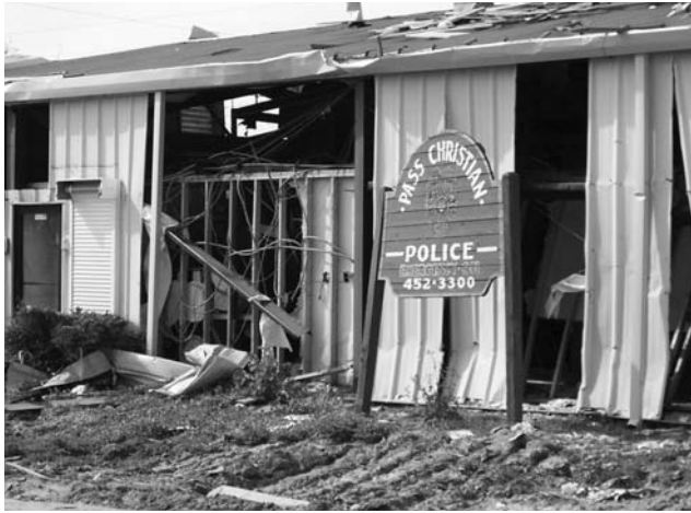
Destroyed Pass Christian Police Headquarters
