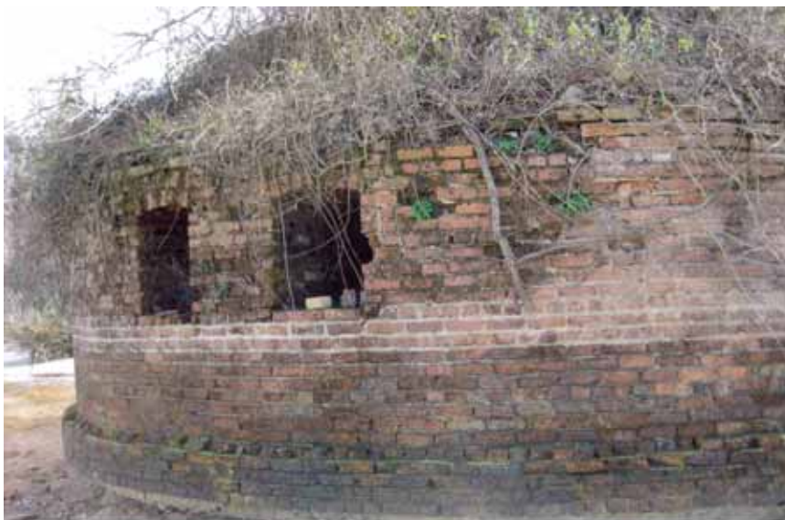
Fig. 1: Brick structure at Ferguson Mill in dry lake bed of Lake Marion. (Photo courtesy of Jim Welch)
